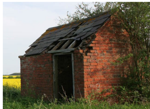
weakened brick wall structure
