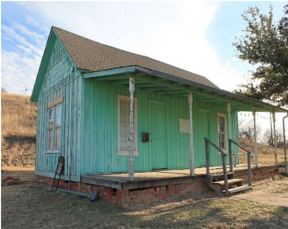
weak wooden frame with wooden panels
