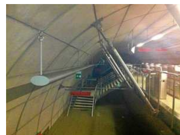
FIG.10 Photographs of damages
