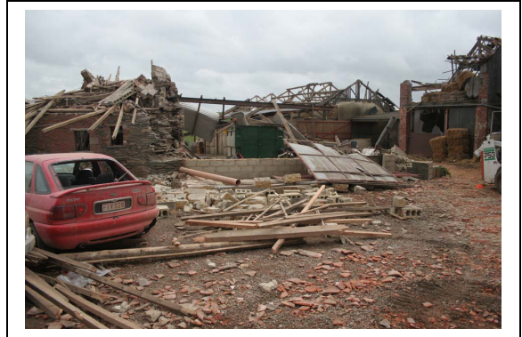
FIG. 4: Damage caused by the tornado shown in Fig. 3 (photo: K.Holvoet)
